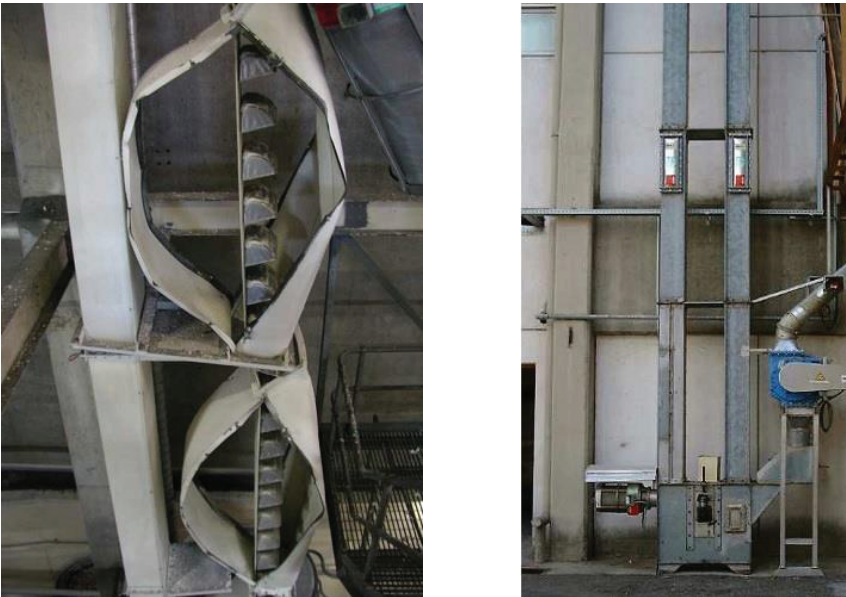
Fig. 6. Example for unprotected (a) and protected (b) explosion harm (elevators)
