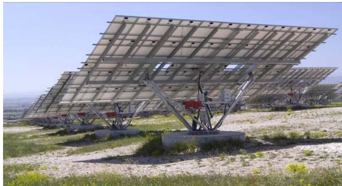
Figure 2.5: MS-2 dual axis solar tracker for 13 kWp [9]
