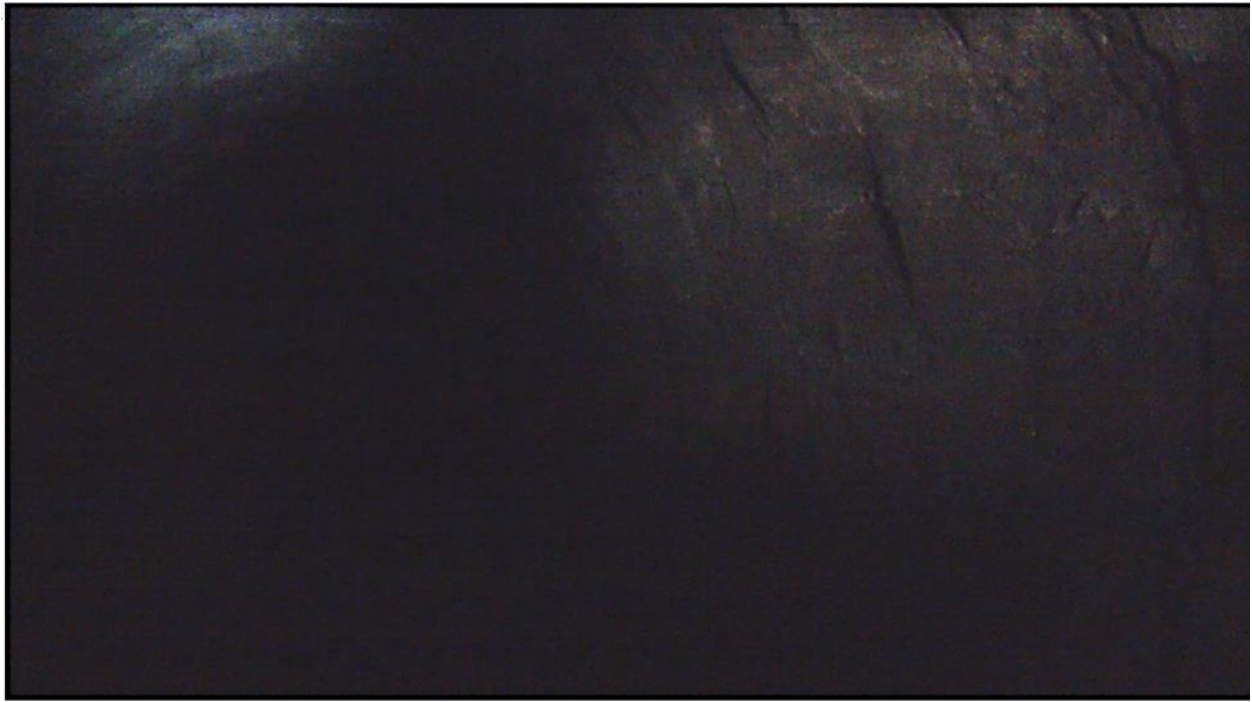
Figure 27 - Screenshot of well #2 footage showing brick lining
