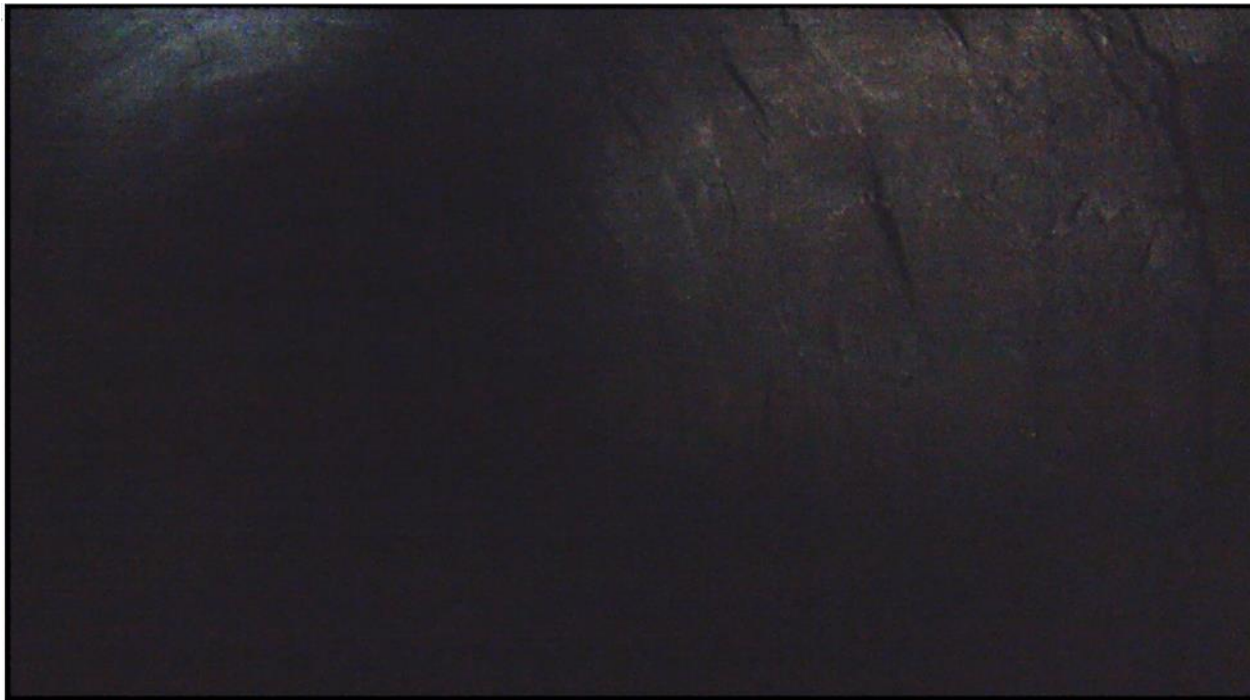
Figure 5 - Screenshot of well #2 footage showing brick lining
