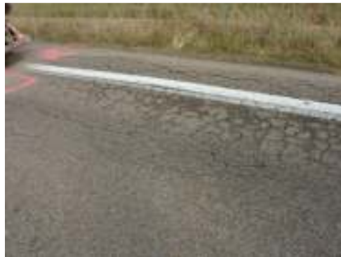
Figure 4.34. Alligator cracking in the outer wheel path of Section 13W.
