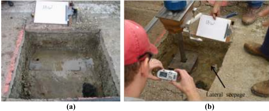
Figure 4.35. Lateral seepage observed in subgrade of Section 13W a) after DCP testing and b) after completion of CBR testing.
