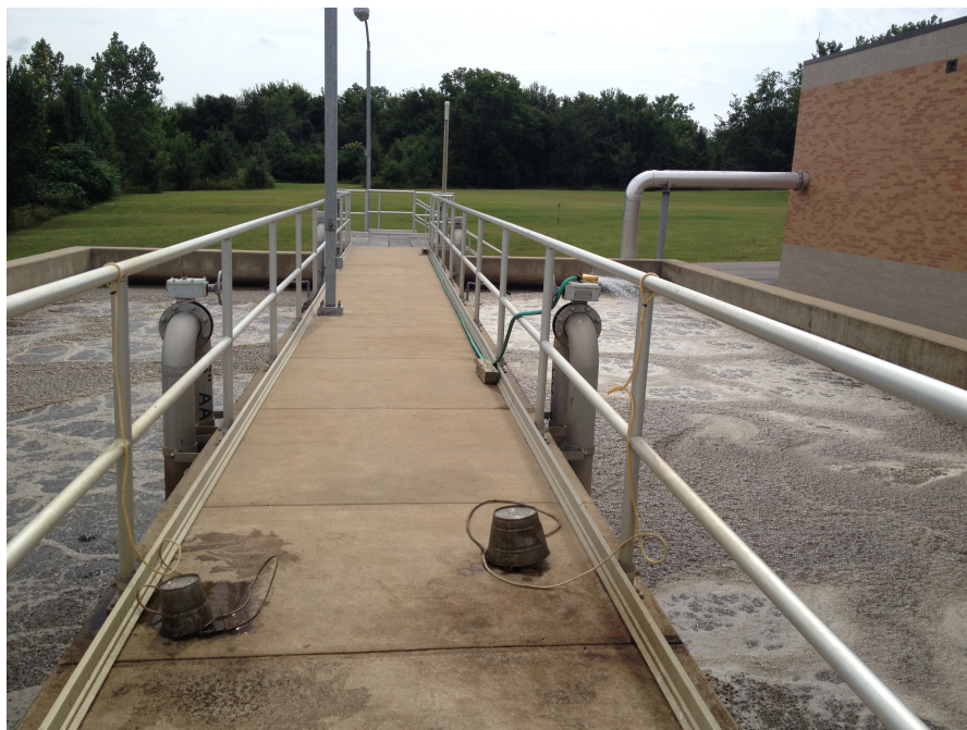
Figure 3: Supplemental Activated Sludge Basin at Massard Plant
