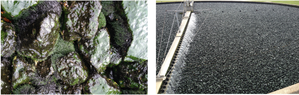
Figure 1 and 2: Trickling filter at the Massard Wastewater Treatment Plant (WWTP) in Fort Smith, Arkansas. Figure 1 is a close-up of the rock media with biofilm attached. Figure 2 is a broader view of the trickling filter with dimensions of 100 feet diameter and 8-10 feet depth.
