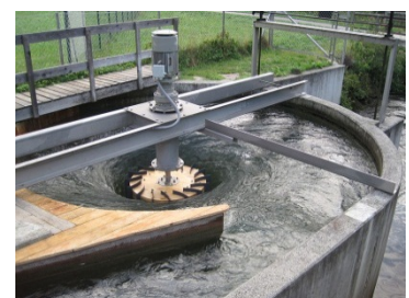
Figure 2 – Vortex Power Generation 4
