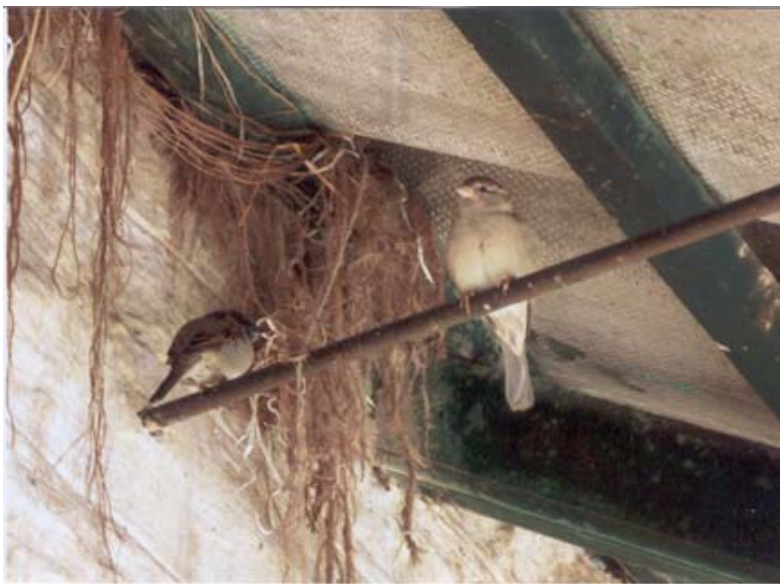
Figure 3. House sparrow nest in the hatched roof.
