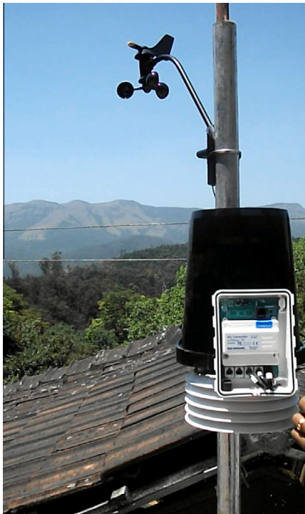
Fig. 19. Photograph of installed wireless Weather Monitoring Station.
