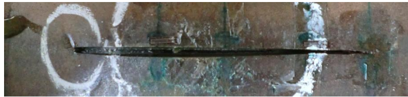
b) Fracture area in SP5-D3-L100
