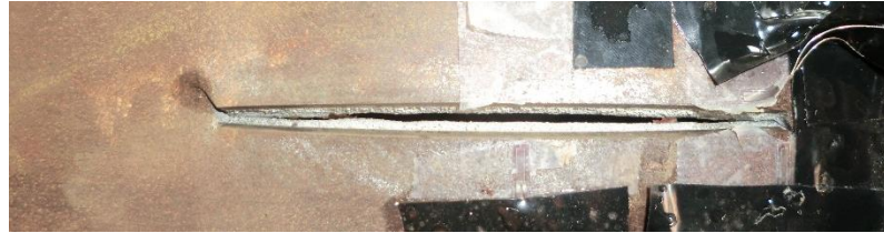
b) Fracture area in SP3-P00-D4
