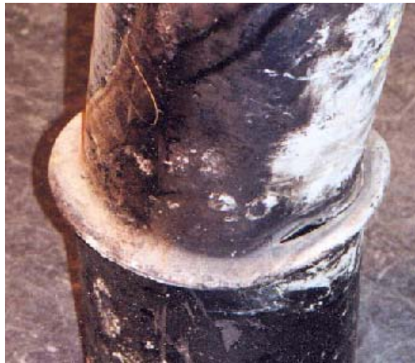
Figure 2.15: Fracture in wrinkle in field NPS10 line pipe (WestCoast Energy Inc.)
