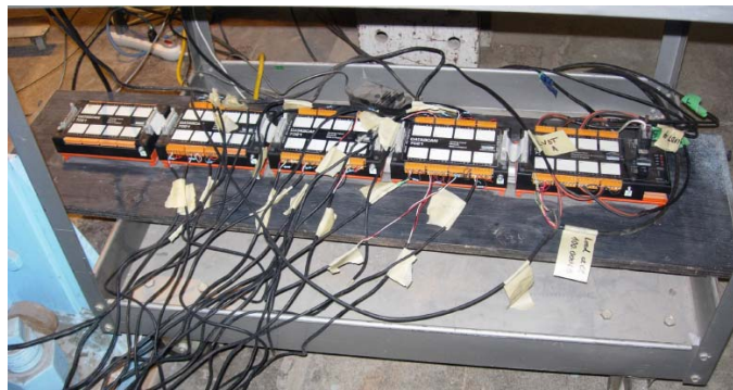
Figure 3.28: Data scan and cable which are connected
