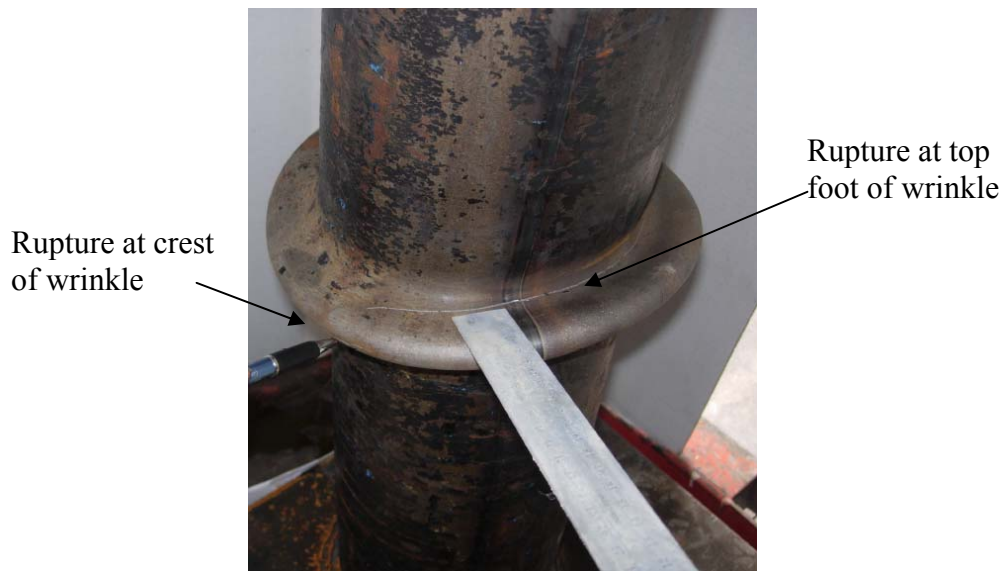
Figure 3.40: Telescopic shape and rupture
