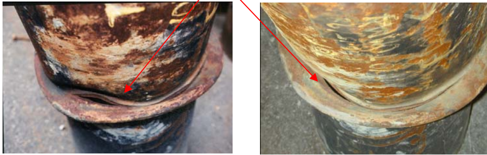
Figure 1.3: Close-up of the rupture in field pipe
