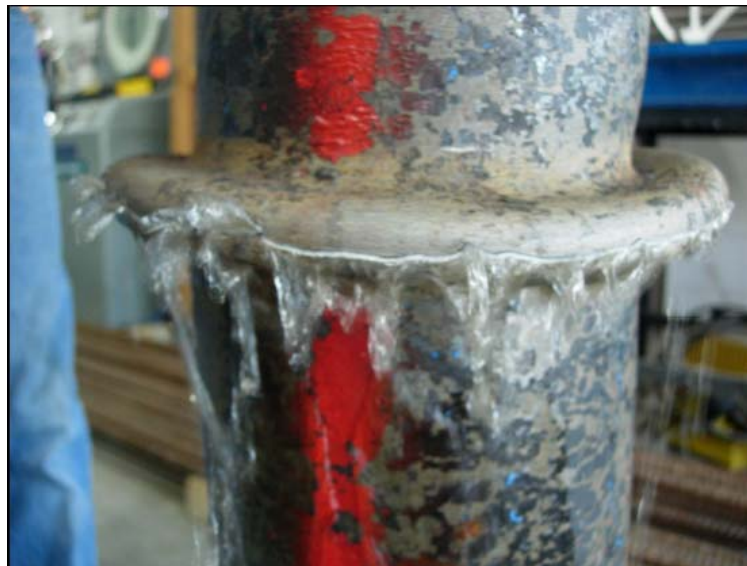
Figure 4.26: Large crack appeared after pressure test
