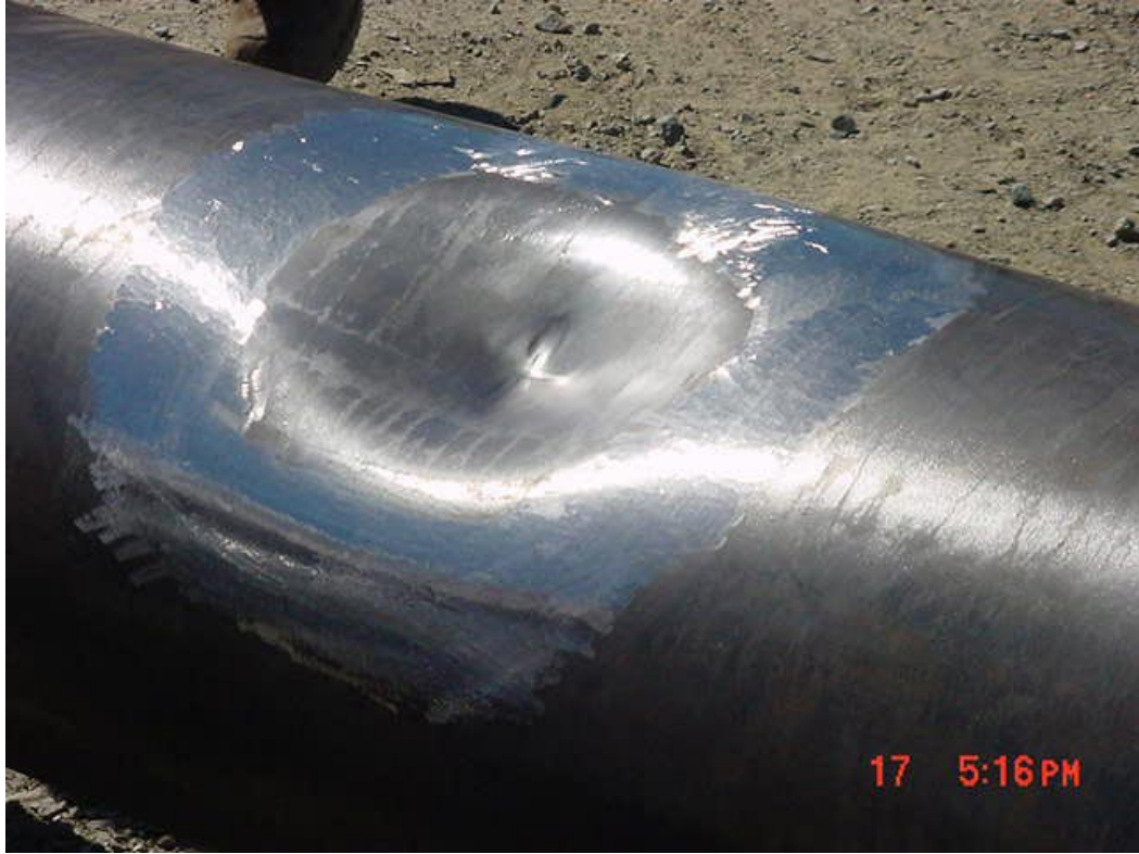
Figure 2.1: Photograph of a dent in the pipe wall (Source: http://www.google.ca/images )
