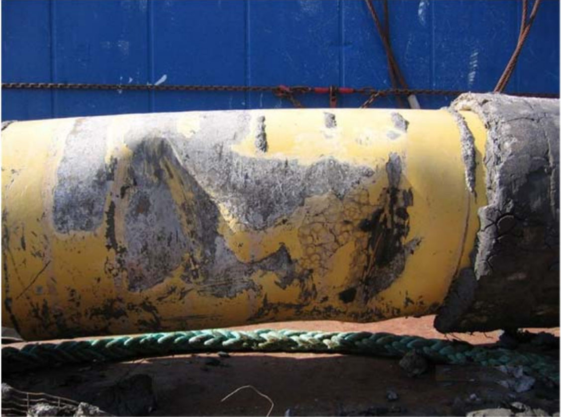
Figure 2.3: Photograph of kinked dent in field pipeline (Macdonald et.al. 2006)
