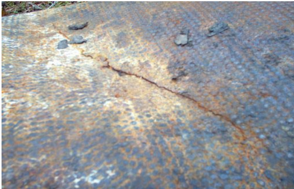
Figure 2.4: Photograph of a dent-crack defect (Source: http://www.easervices.com )
