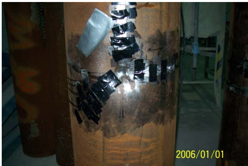
Figure 4.12: Photograph of the dent in specimen SSP20D8
