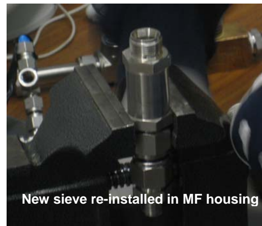
Figure 4.21. Inline micro-filter (MF): (c) Cleaning of filter housing and (d) Filter re-installation.
