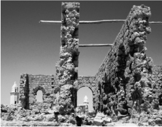
Fig.23 Collapsed building in Suakin
