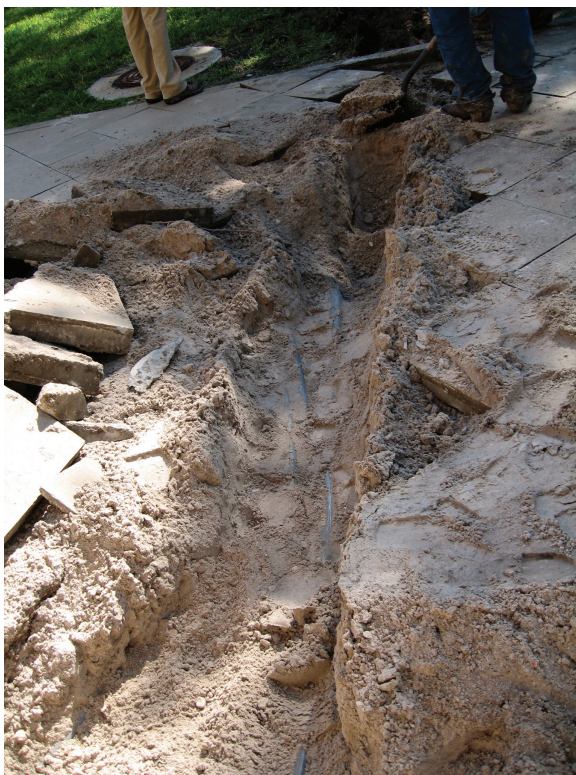
Figure 4-13. Exposed utility lines next to mansion.
