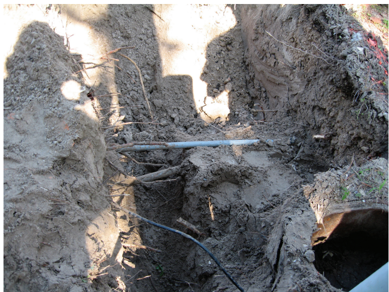
Figure 4-11. Exposed utility lines in Bore Hole A.
