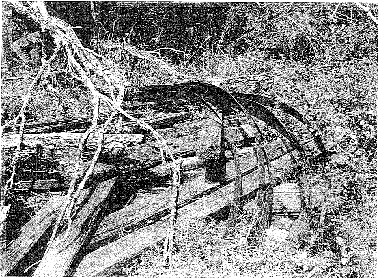
Figure 13-9. Collapsed cypress water tower at 41BX1128.
