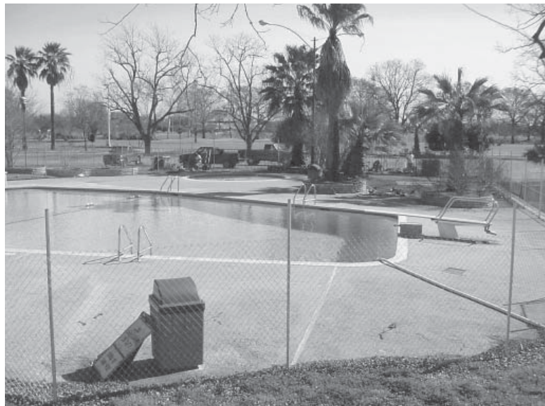
Figure 7-11. Excavations in progress. Unit 4 is in the grassy area by the palm trees in the middle distance and Unit 5 is in the parking lot to the right.
