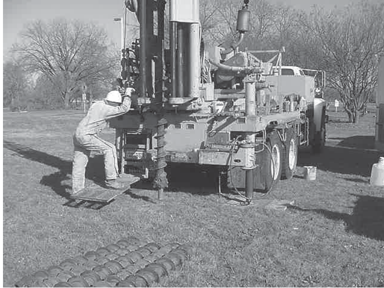
Figure 5-5. Cores were drilled by personnel from the Bureau of Economic Geology, The University of Texas at Austin.
