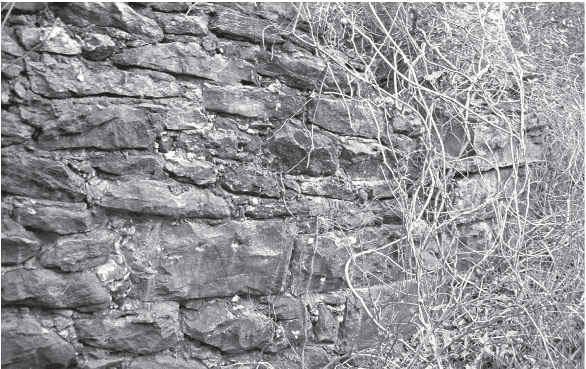
Figure 4-61. Away from the main course of the creek, Aussiloux used smaller sandstone blocks and slabs, with coarse mortared chinking; facing west.
