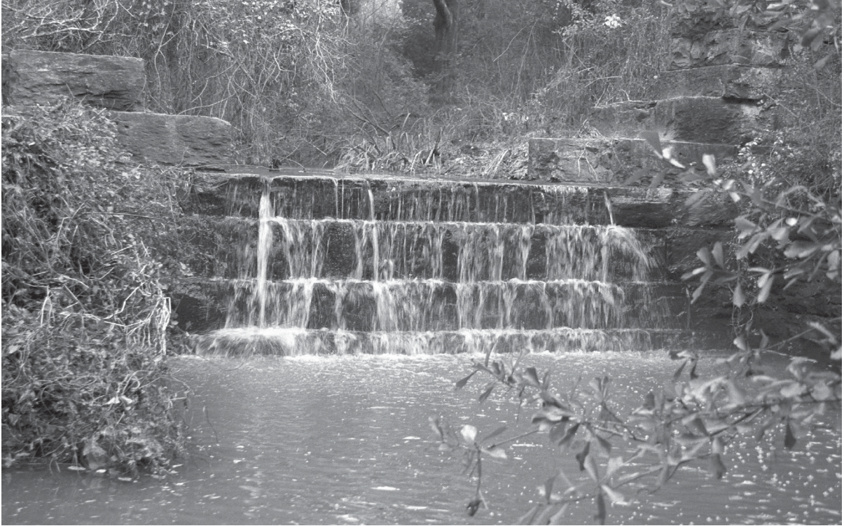
Figure 4-60. French engineer and winemaker Antoine Aussiloux constructed this sandstone dam over Spring Branch (Scott Falls Creek) around 1886.
