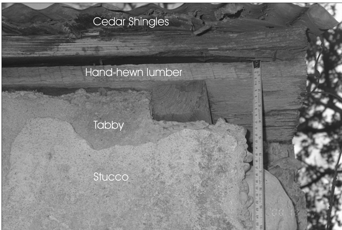
Figure 11. Construction detail of the southwest corner of the stage stop/post office structure, above Unit 3.
