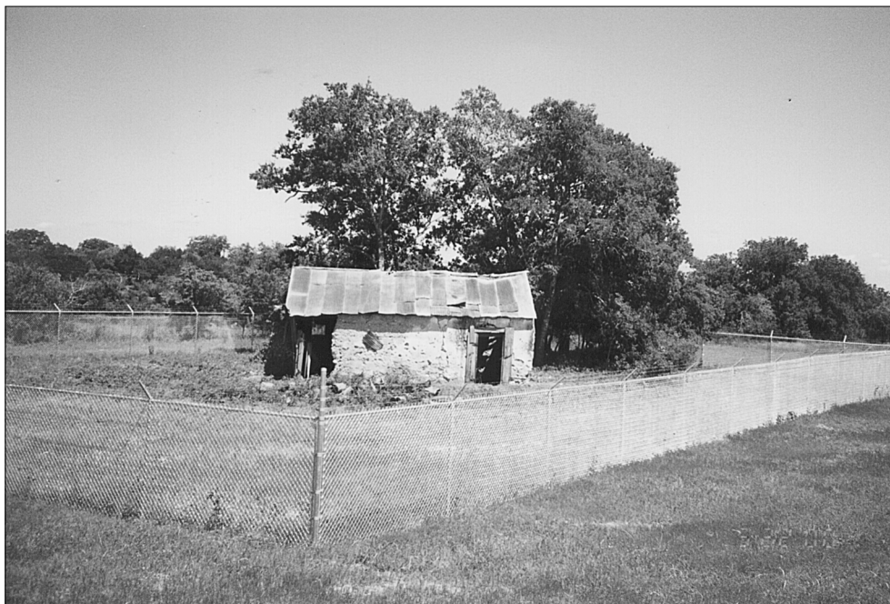
Figure 2. Photograph of western elevation of the Selma Stagecoach Stop and Post Office in 2000.
