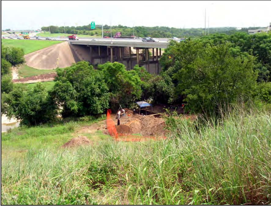
Figure 1.3. Overview of Siren site during early data recovery investigations; facing northeast towards IH 35 and across the river.
