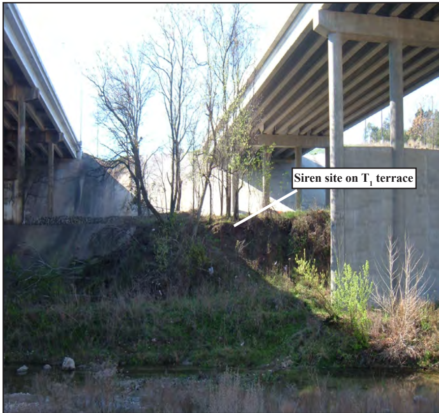
Figure 1.4 Photo shows IH 35 bridge on left and newly constructed frontage road bridge on right, south bank of the South Fork of the San Gabriel River with the river in the foreground, the T_0 and T_1 terraces in middle and T_2 terrace with concrete apron in background; facing south.
