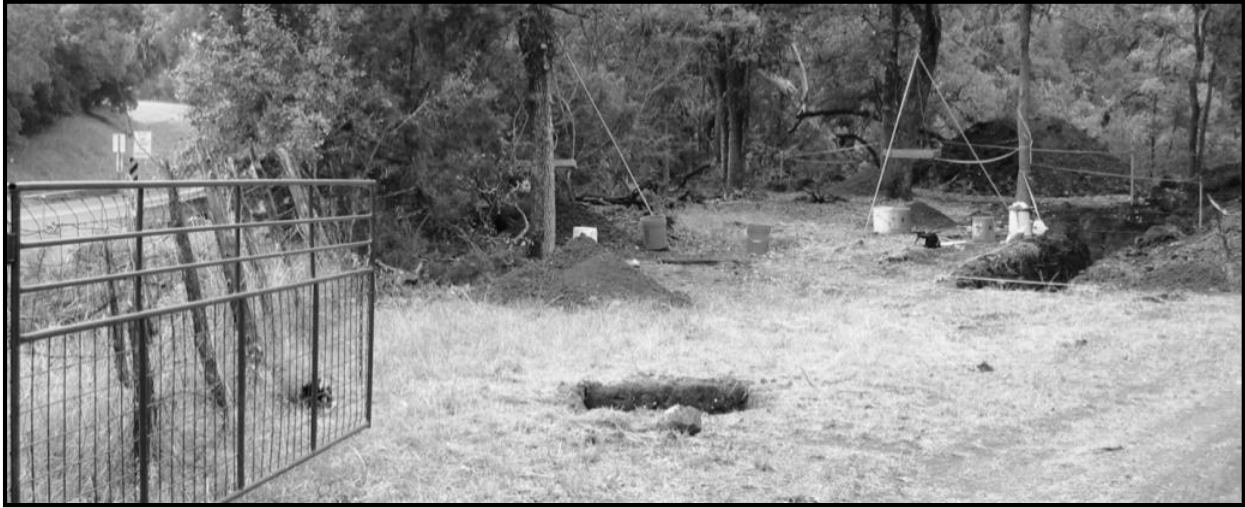
Figure 9-2. View east of proposed easement and east end of terrace with excavation units in progress at 41LM50.
