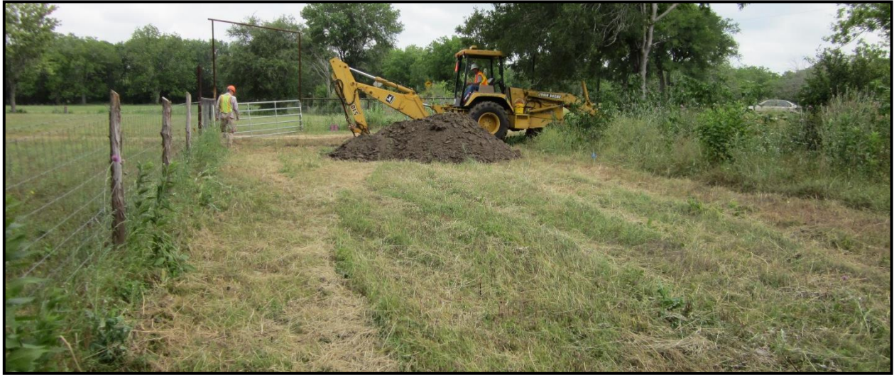
Figure 4-2. Backhoe trenching at northern end of site boundary. New TxDOT ROW fence on left and a buried water pipeline below tall weeds on right.
