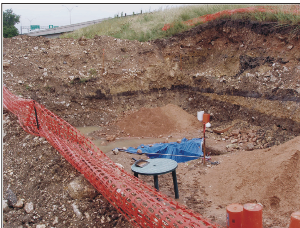
Figure 4-20. Flooding of excavation block during heavy rains.
