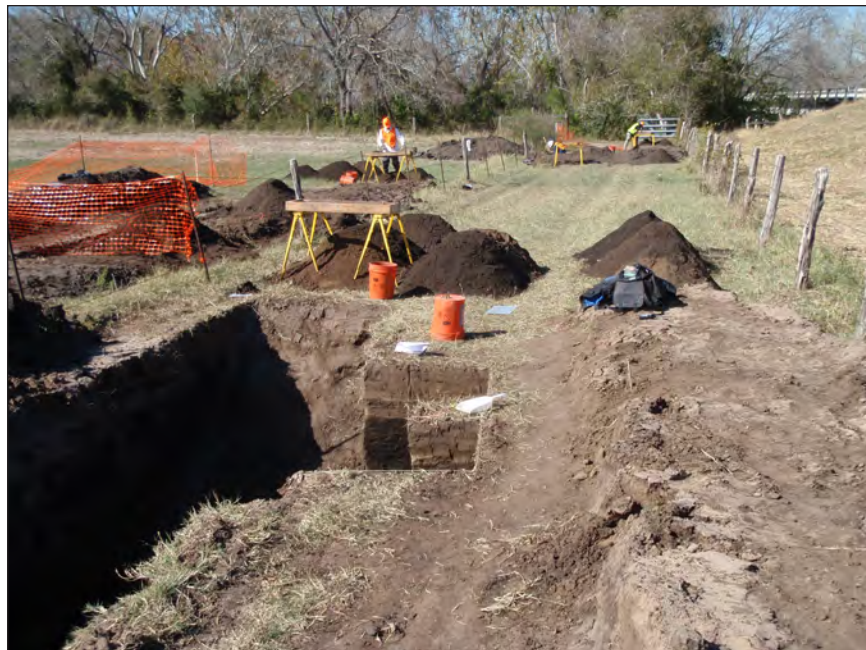
Figure 1-2. View of Site 41DW277 looking toward the US 183 bridge over the Guadalupe River.
