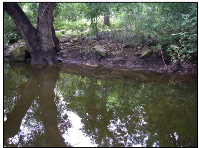
Figure 5.11. Cutbank along Salado Creek on the west side of U.S. 281, facing south.
