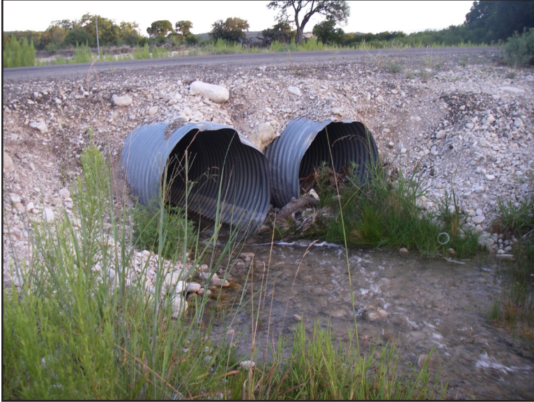
Figure 1.4. Existing tube culverts under FM 2169 at Johnson Fork, just north of the box culverts (facing west).
