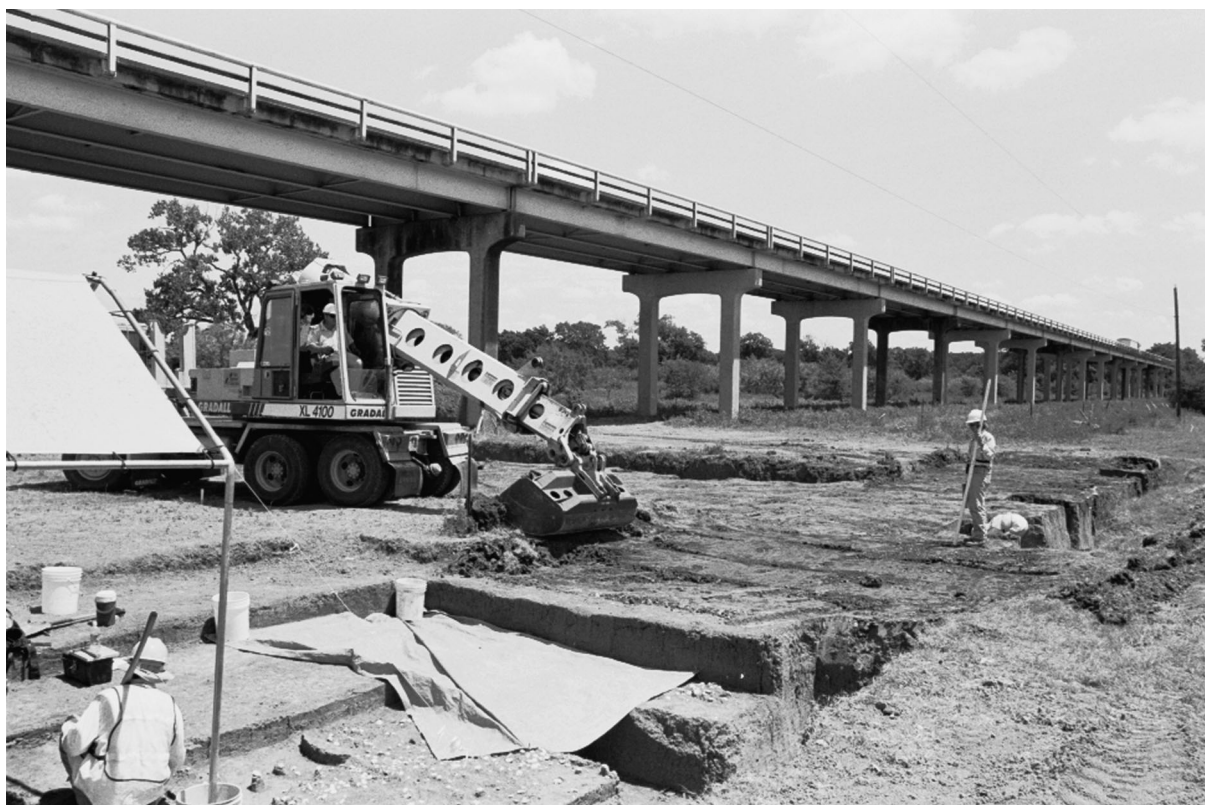
Figure 4-3. View of a TxDOT Gradall stripping the area where the East and South Blocks eventually would be opened as excavations in the Main Block begin.
