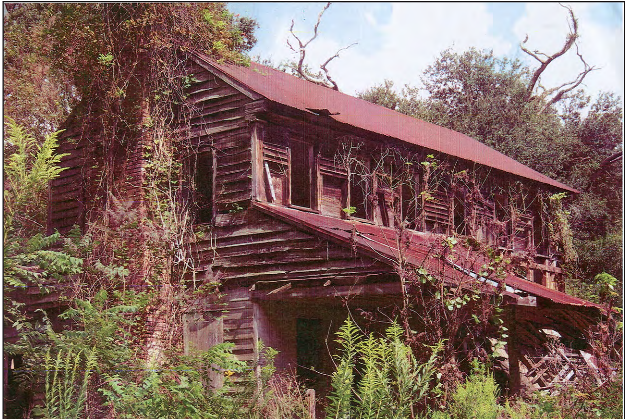
Figure 4-8. View to the northeast of the Taylor/Robert White house, September 2006. The porch has partially collapsed and the interior has been greatly damaged due to the storage of hay in the structure. Compare with Figure 4-7.
