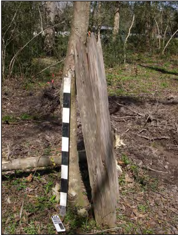
Figure 9-9. Fence post adjacent to Stripped Area 1 at site 41CH371. View is to the northeast. Date: 3/2/07.
