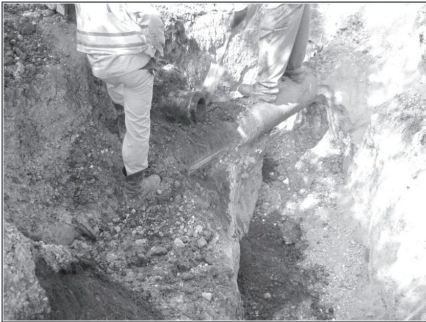
Figure 4-19. Working around old utility lines in a trench on Mission Road near E. White Avenue.
