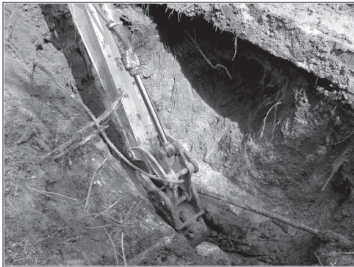
Figure 4-18. Backhoe digging below Mission Road, showing degree of previous disturbance in trench.
