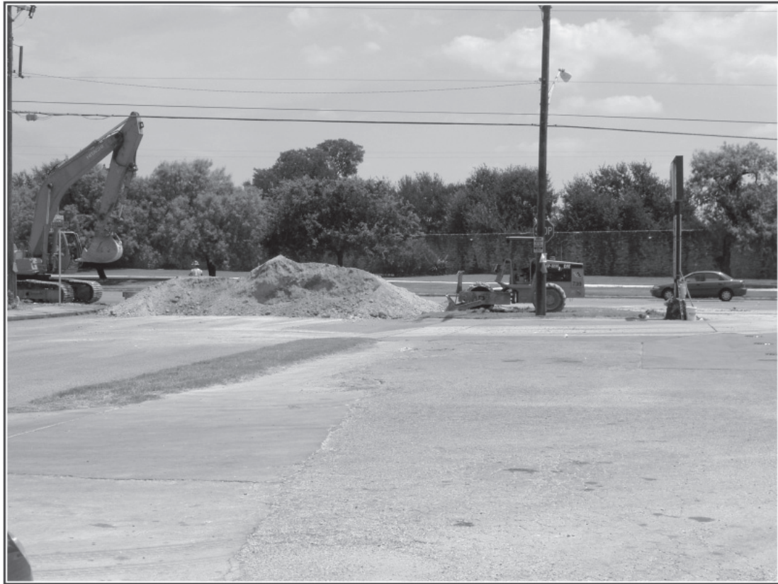
Figure 4-17. Monitoring utility placement on Roosevelt Avenue, looking northeast, with west wall of Mission San José in background.
