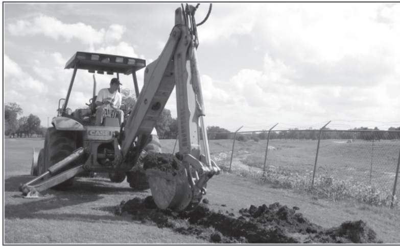
Figure 4-24. Digging Trench C on the north bank of the San Antonio River, near the Mission Road Bridge. Looking southeast.
