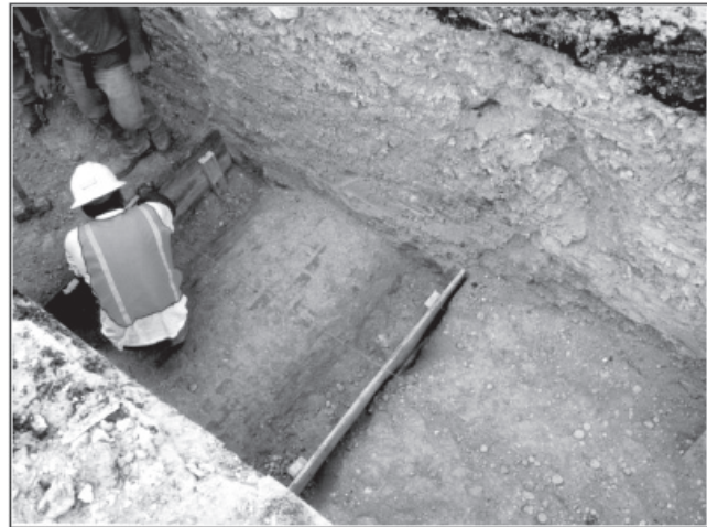
Figure 4-28. Nineteenth century brick sewer line, probably built into the old Concepción/Pajalache acequia ca. 1895-1897.
