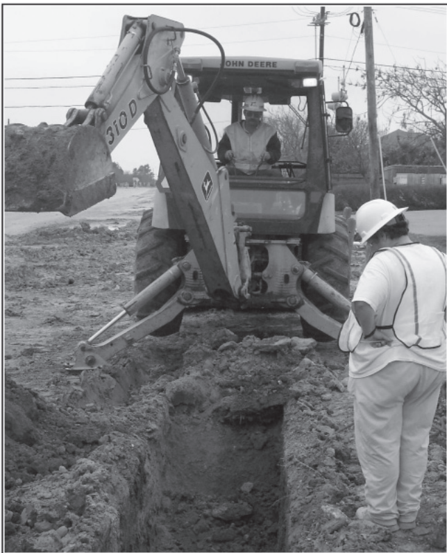
Figure 4-2. Monitoring trench excavation near the location where it is believed Jackson’s 1933 excavations took place. Facing east.
