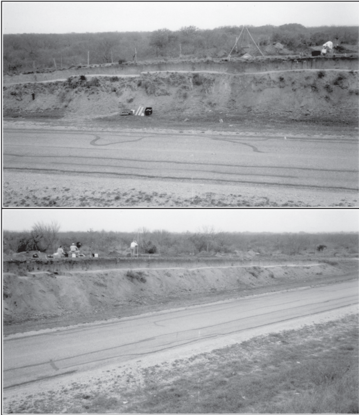
Figure 4-5. Cleaned 75 meter road cut profile. Note dark staining near top and areas of disturbance. Color images of selected sections are available in Appendix A.
