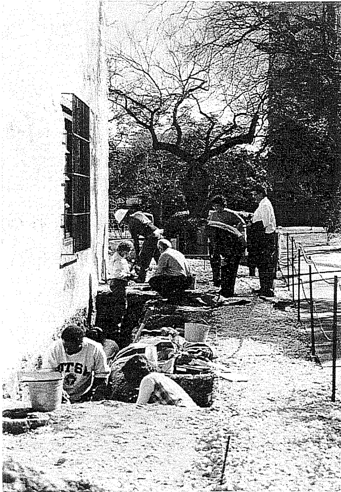
Figure 18. Exterior excavations, looking east. CAR personnel in the foreground are clearing caliche surface by hand while worker shovels near Area B in the background.
