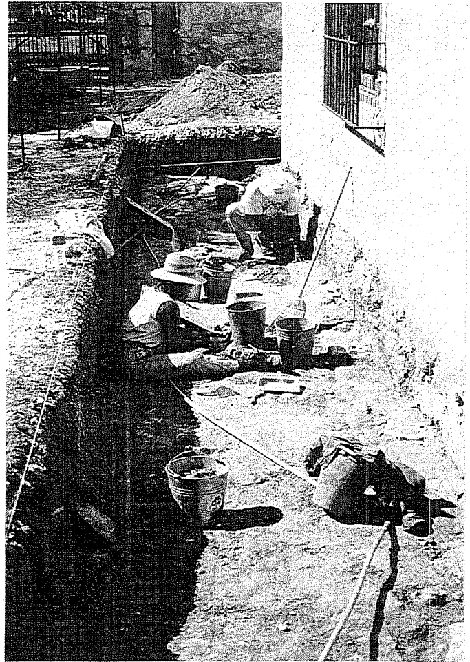
Figure 34. CAR personnel clearing bottom of exterior excavation, looking west. Note the numerous pipes.
