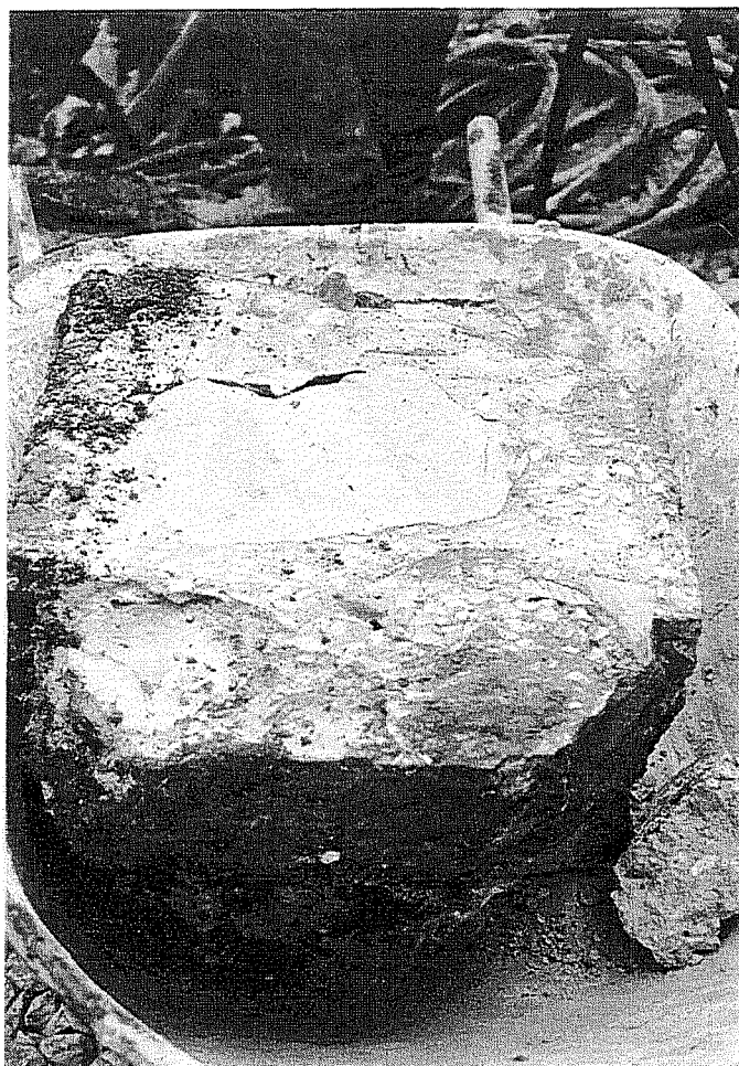
Figure 42. Portion of concrete foundation in a wheelbarrow, during removal, showing cut face. The foundation was 46 cm across. Note the large chunks of limestone.
