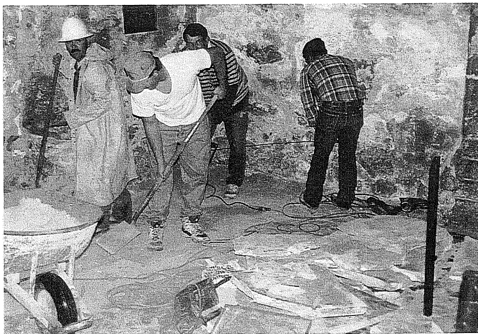
Figure 21. Workers removing the floor on the interior of the south transept. Facing southwest.
