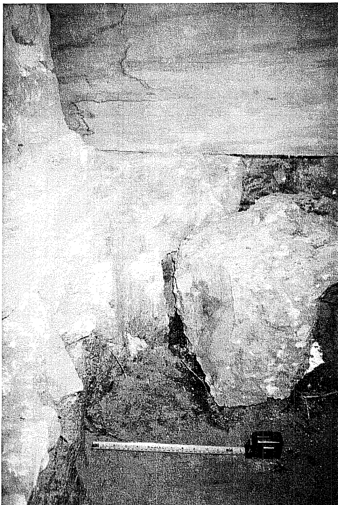
Figure 10. Concrete footing for former gate post at southwest corner of southeast gate.
