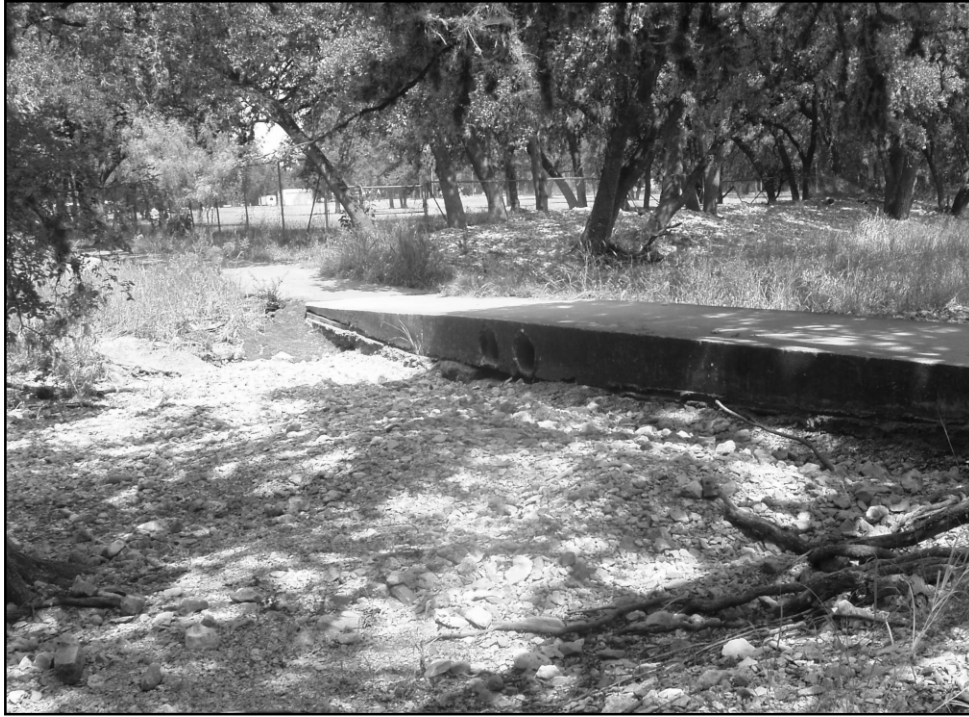
Figure 1-4. Low-water crossing in need of trail repair, Area 2.
