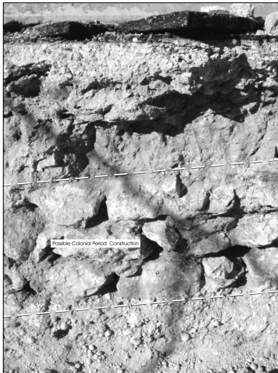
Figure 8-4. Possible Colonial-period wall foundation in the southwestern portion of the project area.
