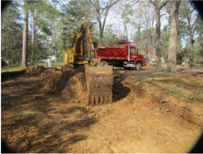
Figure 2. Excavation for PNPC rain garden. Notice the clay soil that has to be removed and replaced by more permeable sands for the filtration to be most effective. Photo by Yanli Zhang.
