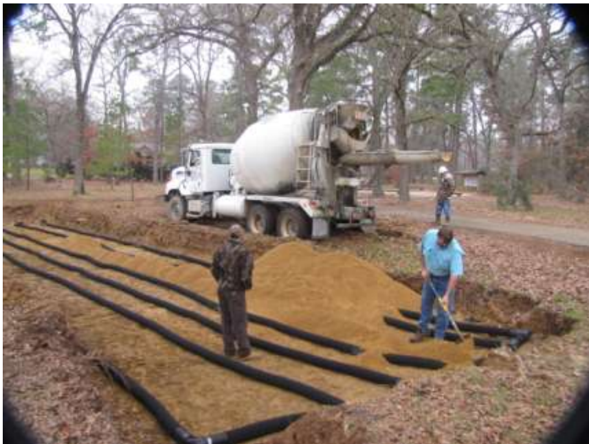
Figure 3. Spreading pea gravel on drainage pipes. The pipes were encased in about 8 inches of pea gravel to allow for adequate drainage, and then were covered by filter fabric. Photo by Yanli Zhang.
