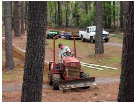
Brad Waguespack operates a ditch witch in the SFA Rec Trails and Gardens to create irrigation lines.
