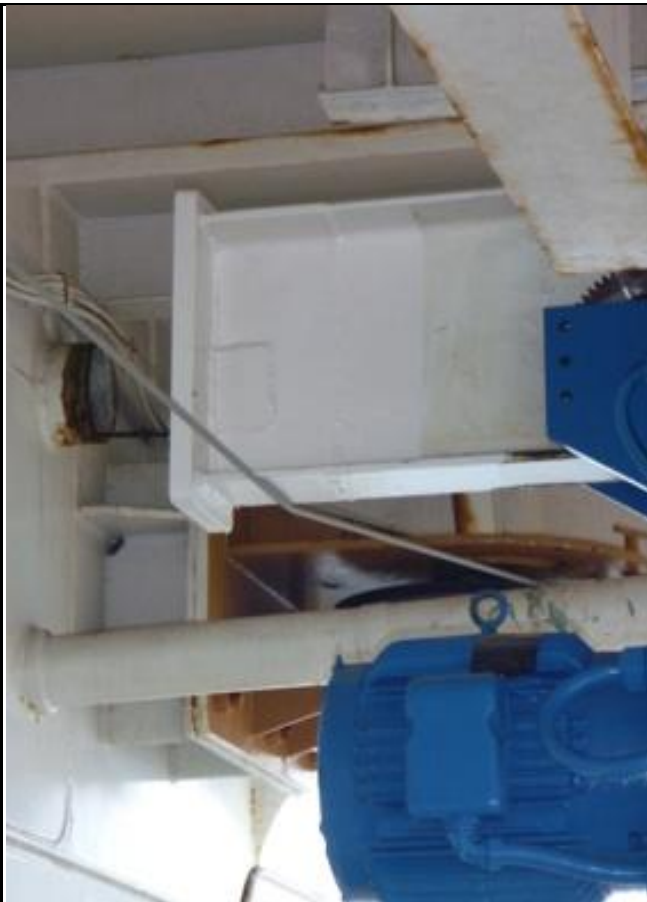
Figure X: CTD wire running over the modified i-beam for the new Shawbox hoist.
