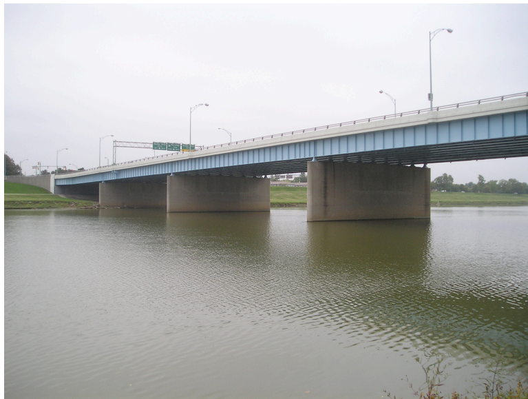
Figure 1. Photo of the Columbia Bridge over the Great Miami River at Hamilton, OH.
