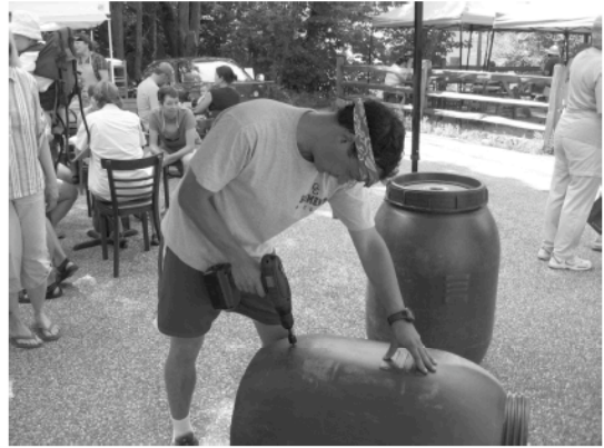
Step 2: Use 3/4" hole saw to drill a spigot hole near the bottom of the barrel
