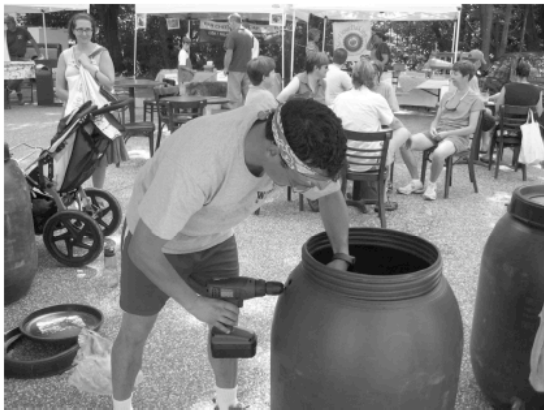
Step 9: Use 1 3/4" hole saw to drill hole near top of barrel for overflow
