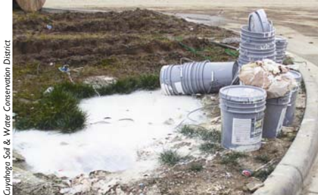
Paint spill at construction site
