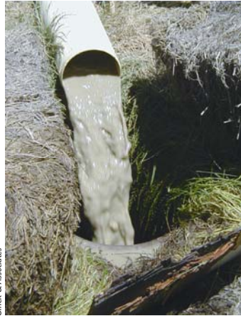
Drainage with heavy sediment load
