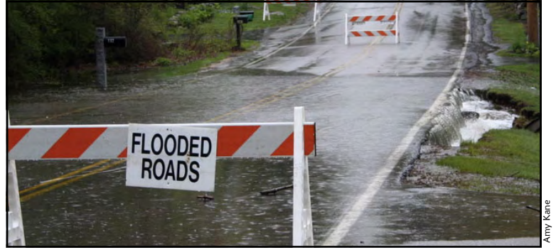
Flooding in 2006 and 2007 damaged property and closed several roads in North Hampton, including Mill Road at the Little River crossing pictured above.
