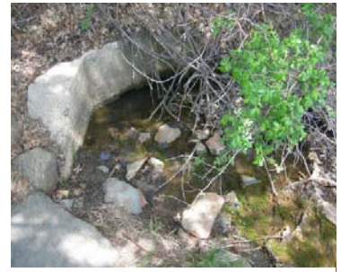
Significant hotspot stormwater outfall in Admiralty Village in Kittery
