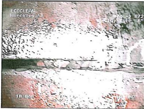
IMAGE: 12b, TAPE #: 11/29/2005 102.9FT, offset joint, slight
