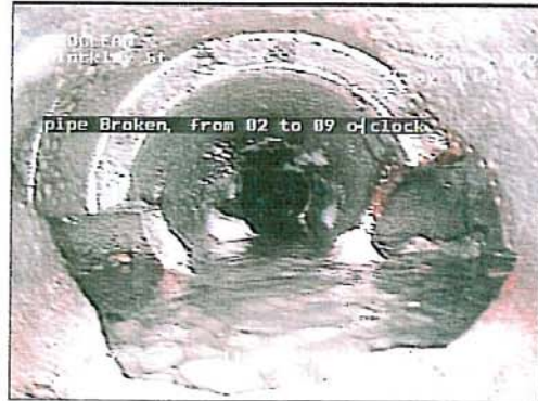
IMAGE: 13a, TAPE #: 11/29/2005 110.65FT, pipe Broken, from 02 to 09 o'clock
