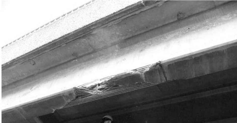
Figure 1.1 – Example of impact damaged bridge girder provided by the Washington State Department of Transportation (WSDOT)
