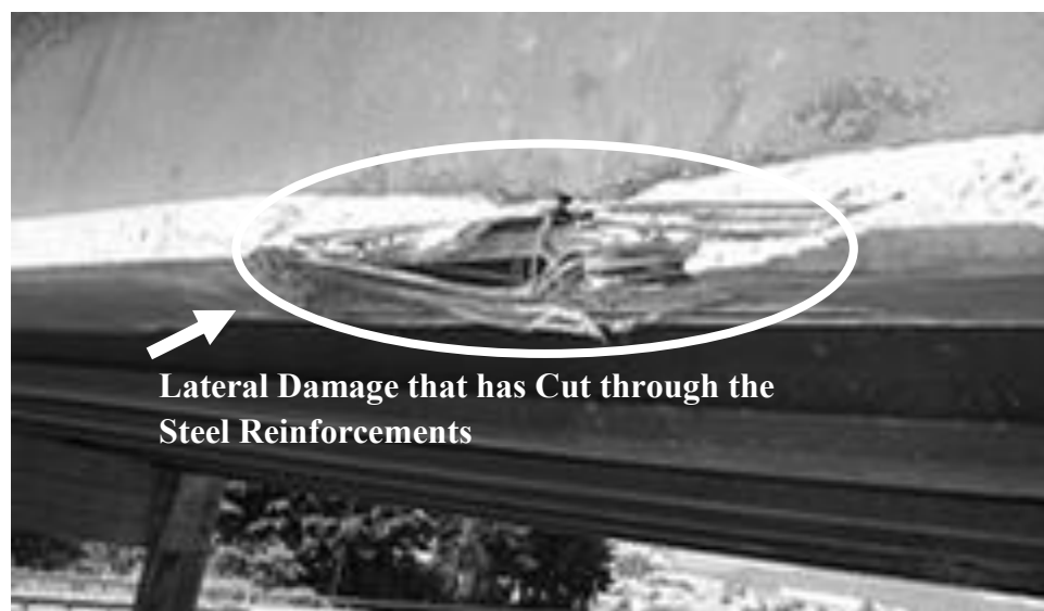
Figure 1-1: Example of overheight impact damage to prestressed concrete bridge girder
