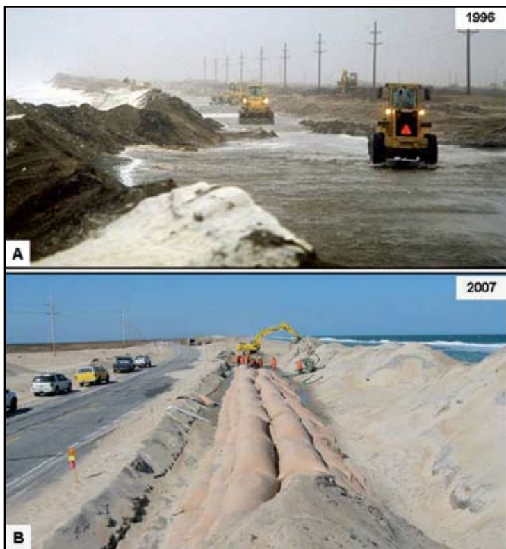
FIGURE 15. Panel A is a photograph that shows NC Highway 12 on Pea Island “going-to-sea” in a 1996 storm. Panel B shows the late 2007 effort to anchor the constructed barrier dune ridge along NC Highway 12 with an internal core of sand bags. Panel A photograph is from Pilkey and Thieler (1992). Panel B photograph is by D. Stewart, Pea Island Wildlife Refuge.
