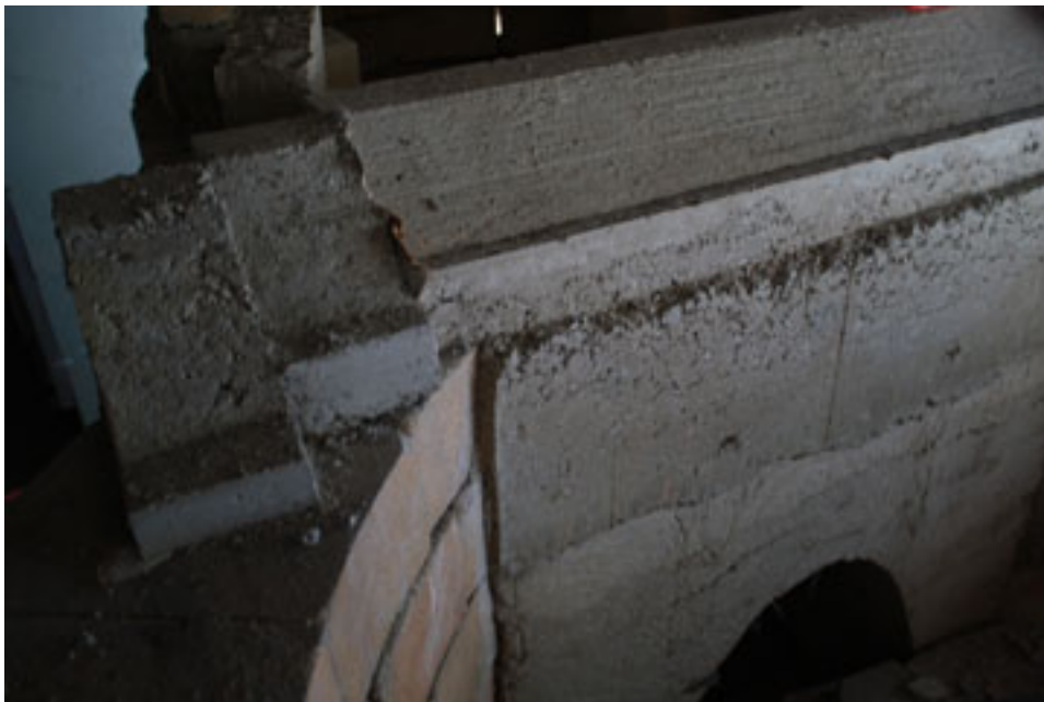
Photo 4 – Castable skew bricks
