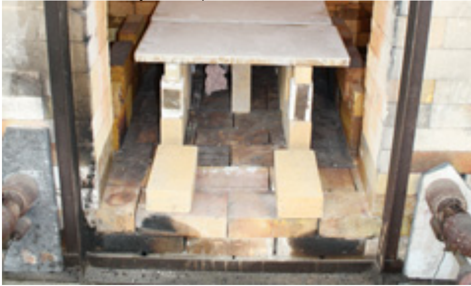
Photo 5 – Secondary burner ports built into door
