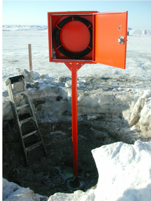
Figure A.5.: Steel box for the protection of the surface ends of the DTS cables on the Mallik 3L-38 well, Mar. 12, 2002.
