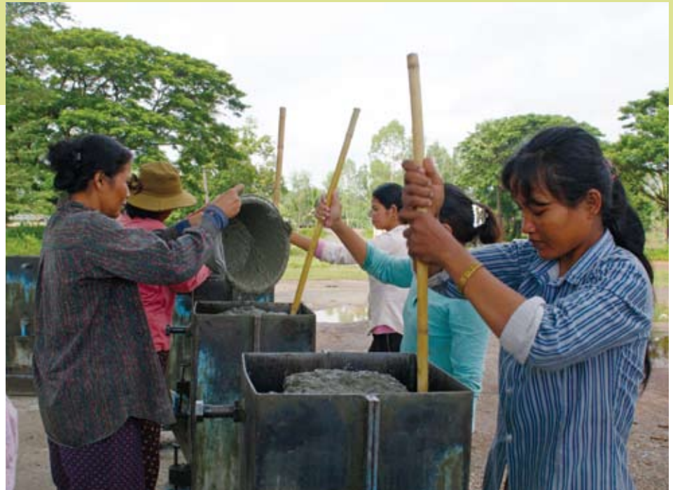
Families play a role in producing their own filter, here filling the mould with concrete.
