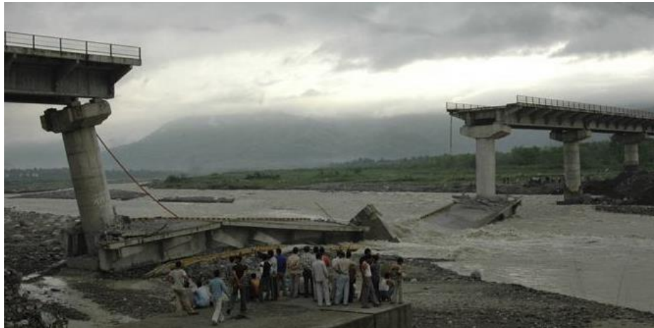
Foto 2-2 Colapso de (Nalgonda District Bridge) near Veligonda-India Fuente: (Diario The Caravan, 2005)
